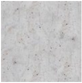
Masonry Concrete Stained QP29
