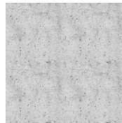
Masonry Concrete Splintered
