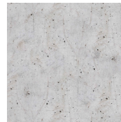
Masonry Concrete Stained
